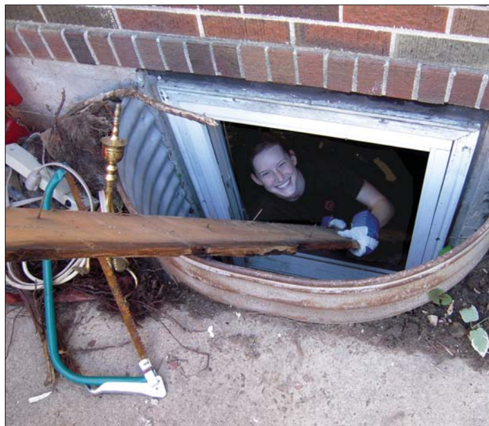
WI Grad chapter vice regent Lisa Vanevenhoven helps remove rubble from the basement while remodeling the WI Grad-Beta Psi chapter house.
